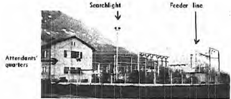
Overall view of a transformer station
