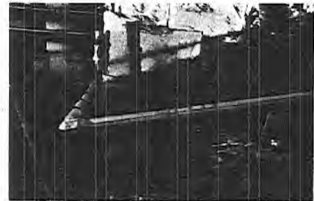
At the bridge support, the cable comes out of the ground, crosses over the water along the bridge and then reenters the ground on the opposite bank.
