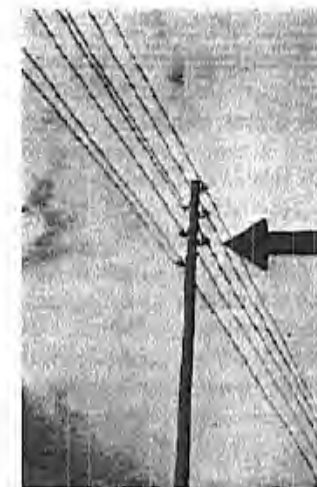
High tension wire Insulators are staggered
