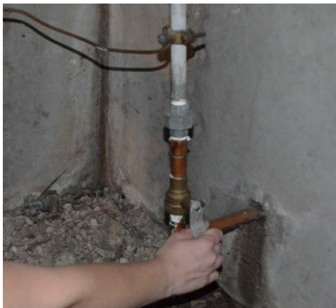
Locate the shut-off valve where the water line enters the house.
