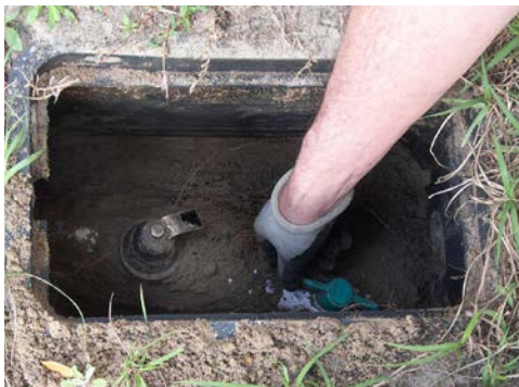
Water can be shut off to a home or a commercial building by locating the water meter outside, often in the ground in front of the structure.
